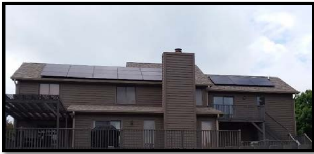
Note: a roof mounted solar energy system located on the rear of a home or accessory building and installed in a uniform pattern is permitted as a matter of right.
