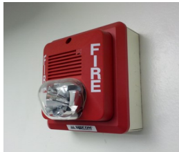
A FIRE ALARM SYSTEM MUST BE INSTALLED IF THE BUILDING DOES NOT HAVE ONE.
